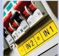
Distribution boxes & patch panels
